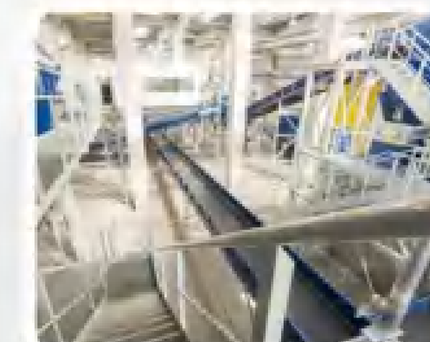
Total system visual monitoring
