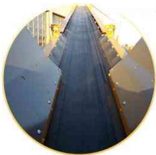
输送带 Main conveyor belt
